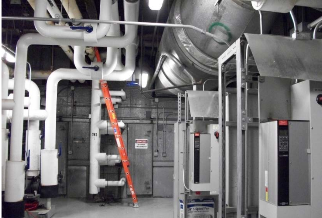
Figure B-0-9: One mechanical room view
